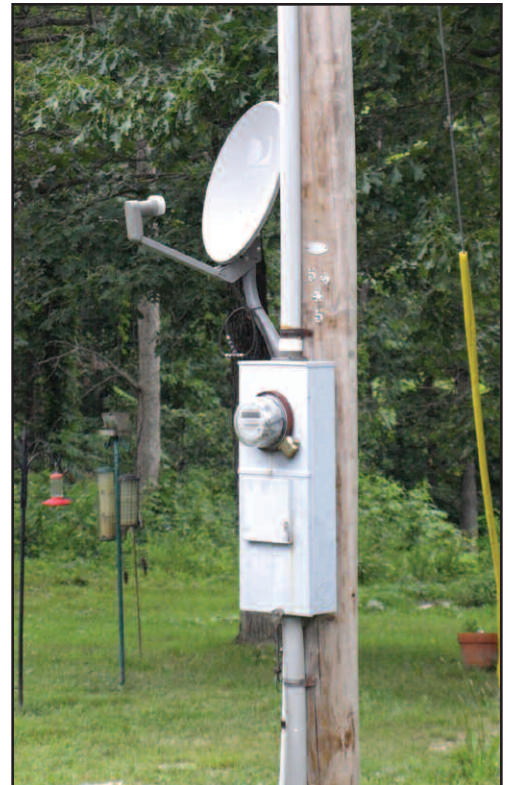
Satellite dishes and other unauthorized attachments must be removed to protect lineworkers.
